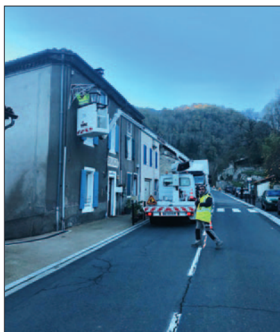
Installation illuminations Noël.
