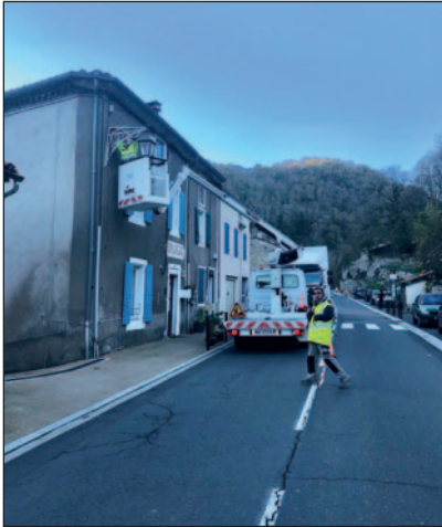
Installation illuminations Noël.
